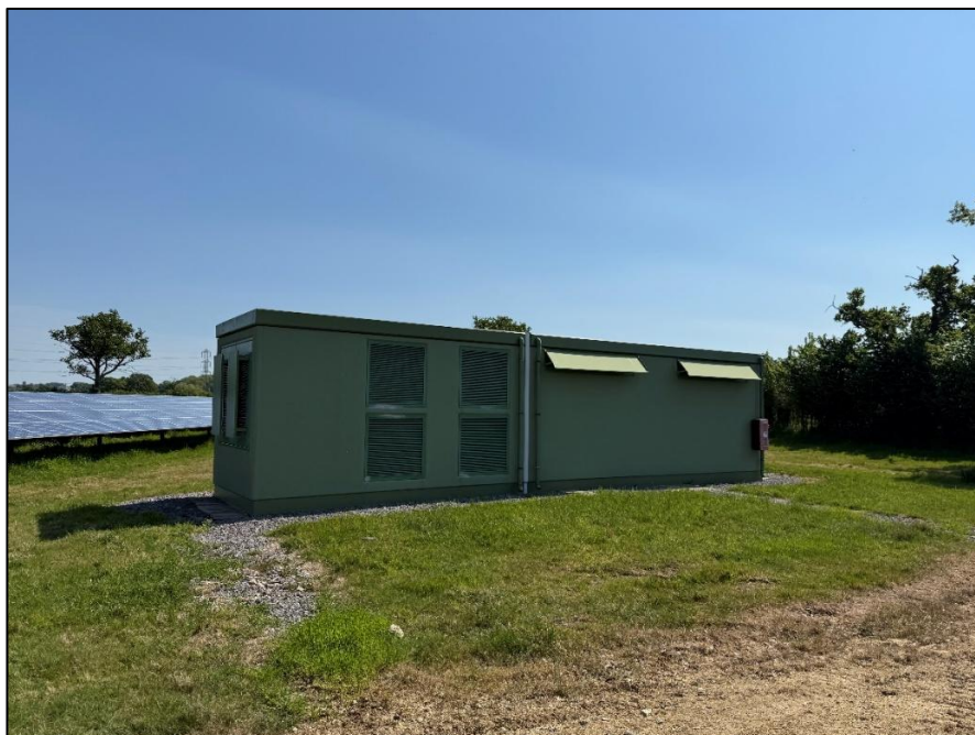
Plate 6 Typical Conversion Unit / 33kV Sub-distribution Switch Room
