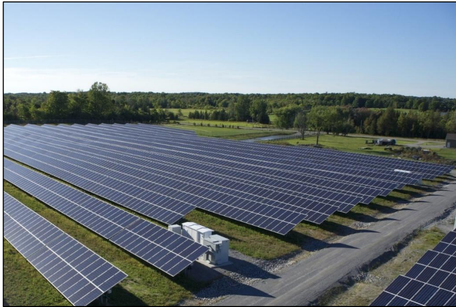
Plate 5 Typical Fixed South Facing Arrays (with Conversion Unit/Inverter) 33kV Sub-distribution Switch Rooms
